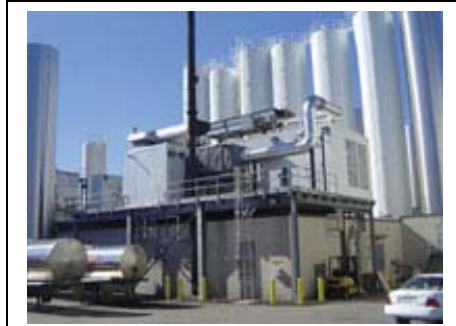
A two megawatt co-gen system recently came on line at Dean Foods' Garelick Farms plant in Lynn, MA. Outside investment paid for the project. Source: EPS Corp.
